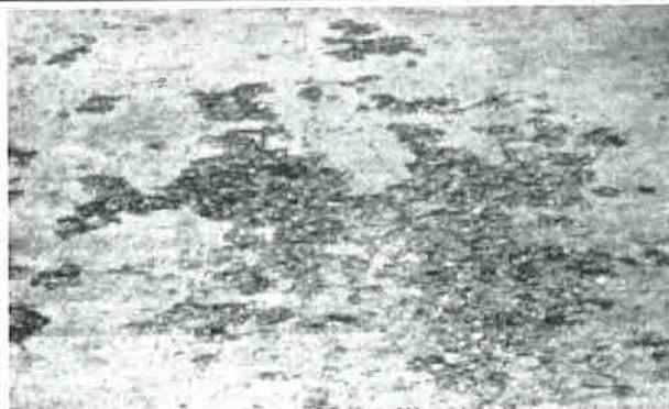
Scaling concrete surface
